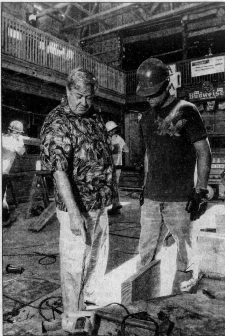
Flora-Bama Lounge & Package co-owner Joe Gilchrist, left, and construction foreman Nick Swan discuss progress Wednesday at the "Bama-Dome" portion of the establishment that is currently being renovated. BEN TWINGLEY/BTWINGLEY@PNJ.COM
